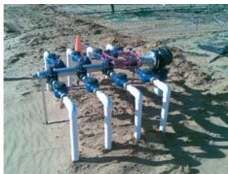
Flow meters for eight irrigation treatments at Lake Powell
